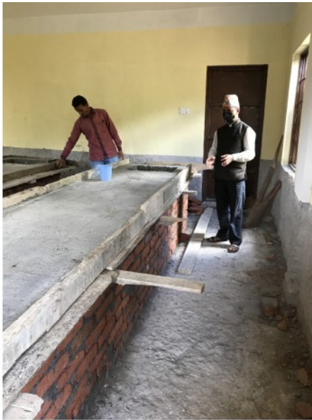
Above: Building the lab benches in the new science lab at Sunaula School in Nepal.
